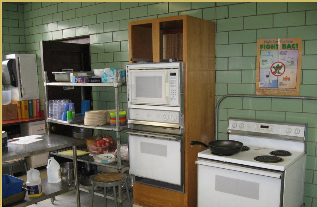
Kitchen in need of renovation
